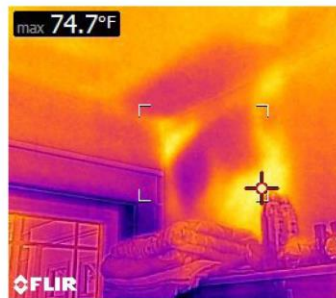
Missing Insulation – Summer Day E6 with MSX
